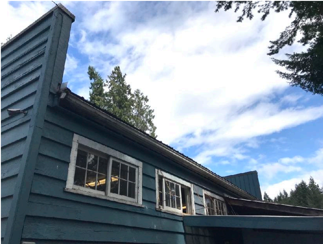
view of the roofline off the store exposition showing the false fronts, front and rear.
